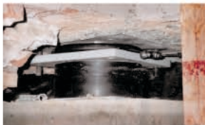
RS 400 over lead-rubber seismic isolator, Campbell Hall, Monmouth, OR
